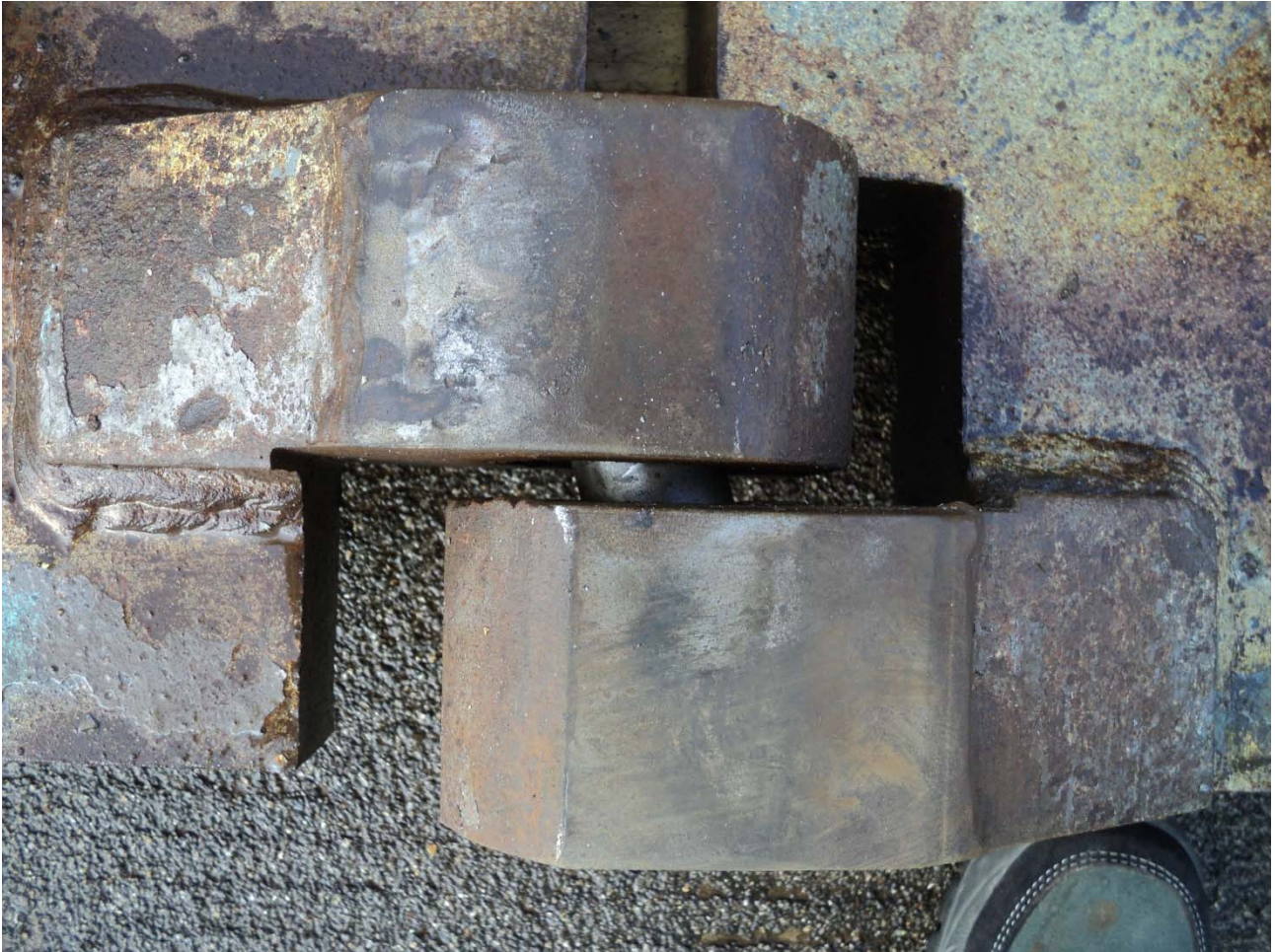
Photograph 14 – Excessive wear on hinge, gap opening between joints and hinge pin lateral rotation.
