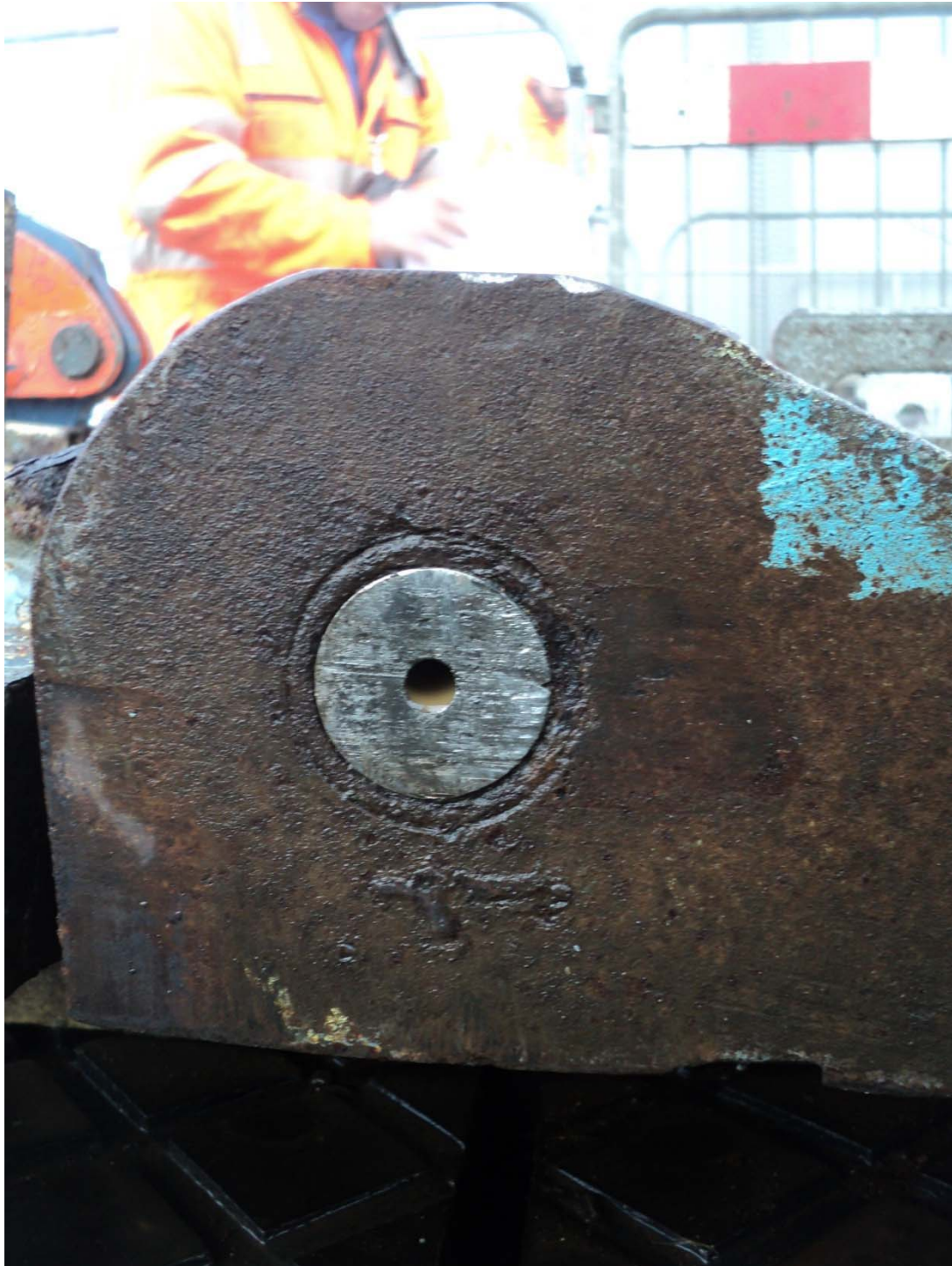
Photograph 2 – Hinge at extreme end of Joint showing original condition of hinge pin and foot profile (note foot profile is slightly flattened).
