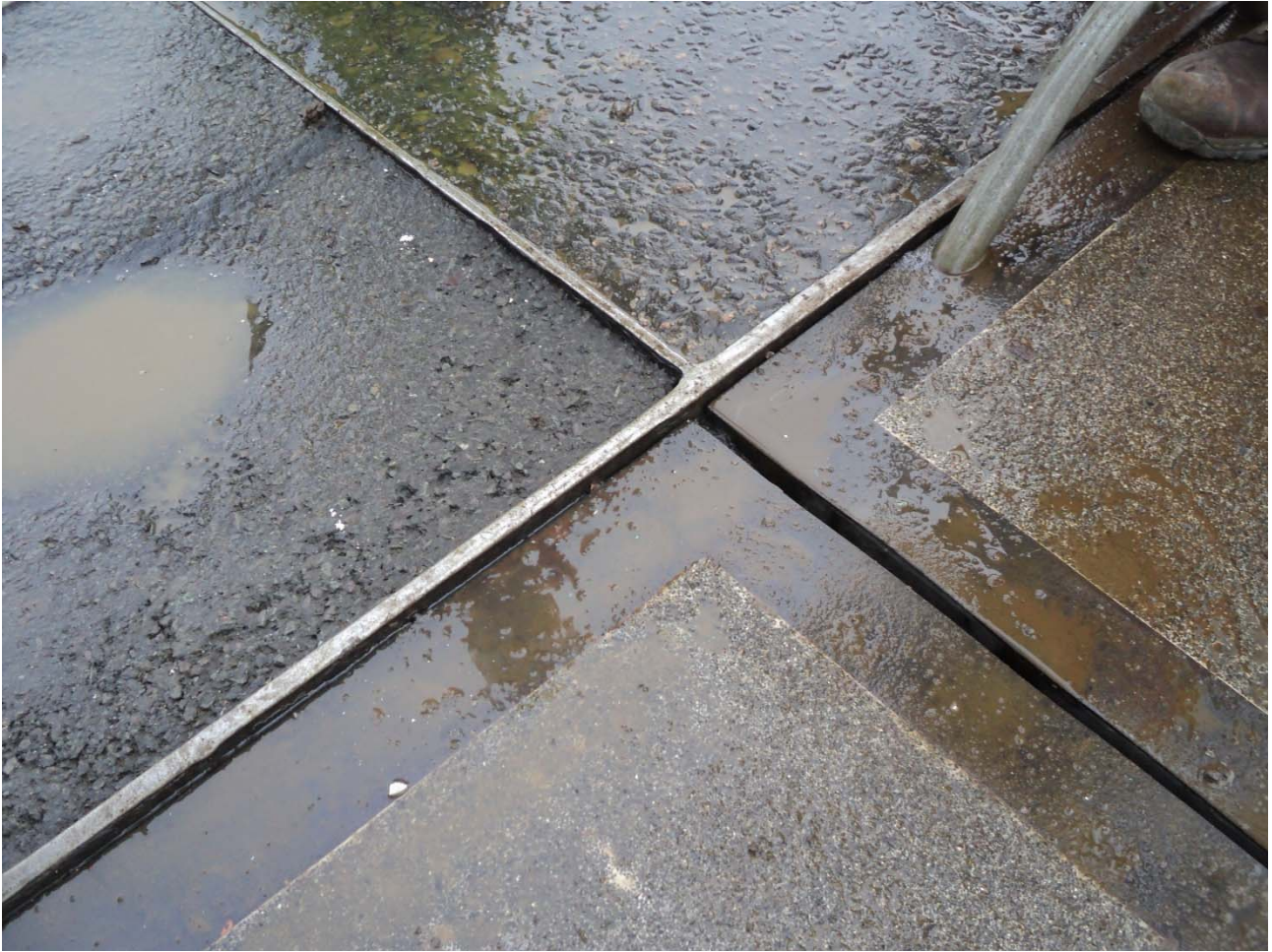
Photograph 8 – Worn edges and uneven ride surface. Note drop in joint level due to wear on bearings.
