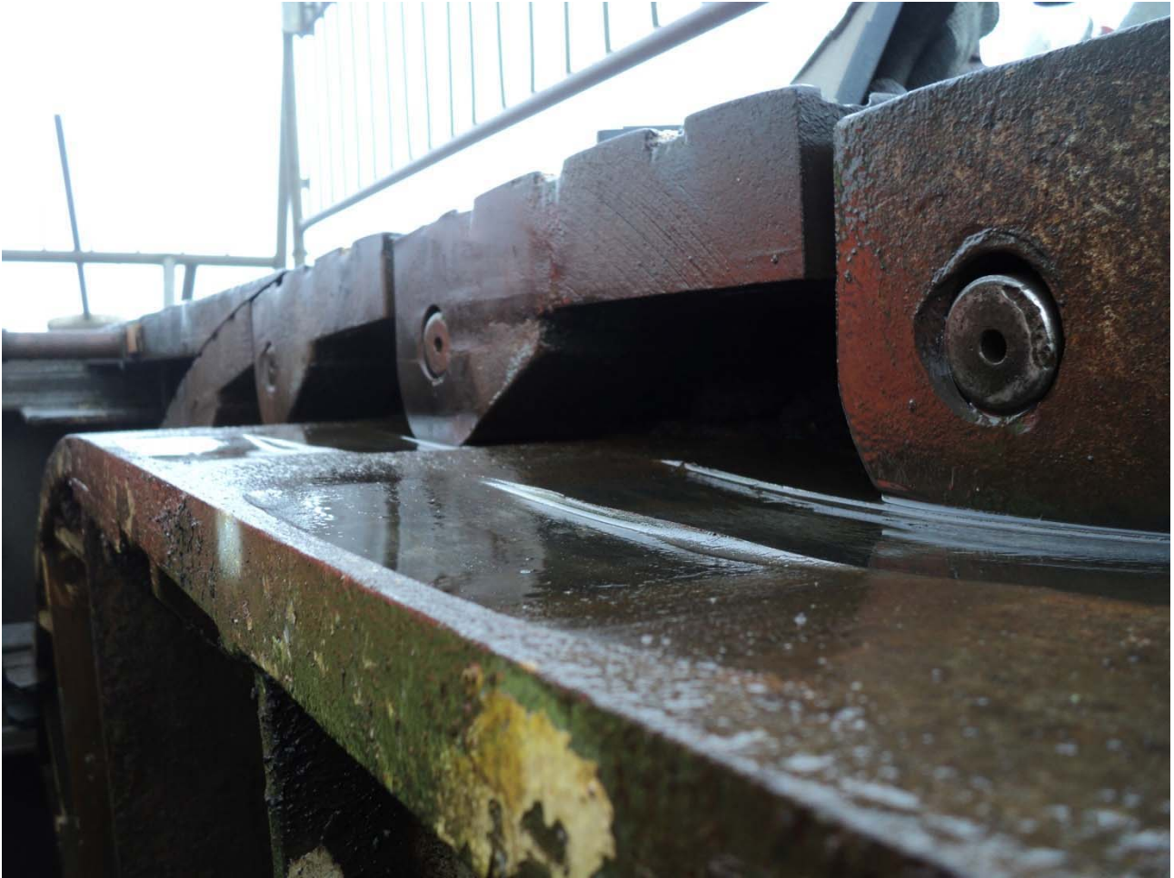
Photograph 11 – Wear in slide track at typical hinge positions. Note uneven carriageway level.
