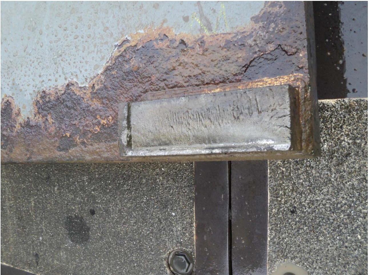
Photograph 7 – Worn anchor plate bearing.
