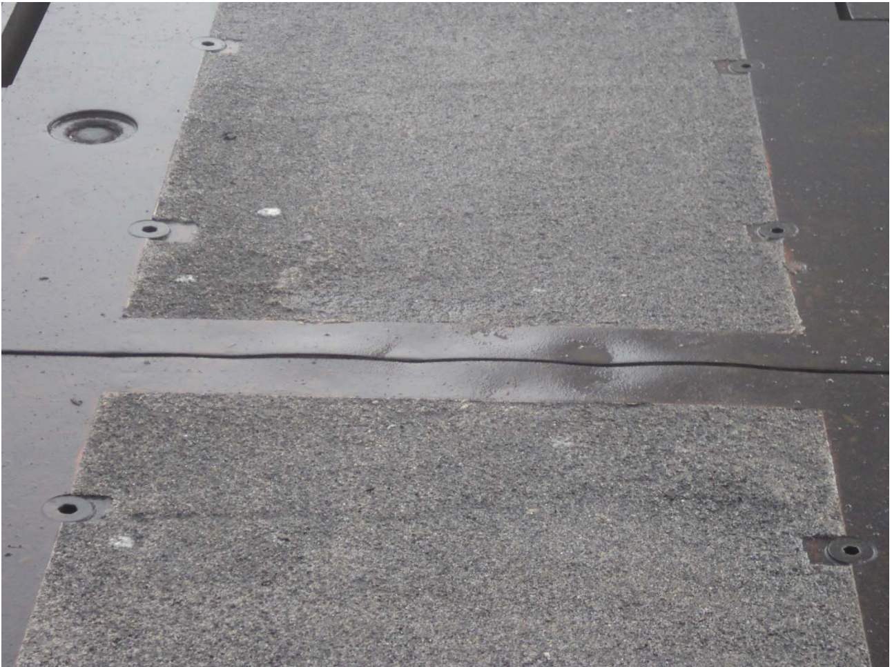
Photograph 19 – Rippling in edging steelwork to carriageway surfacing.
