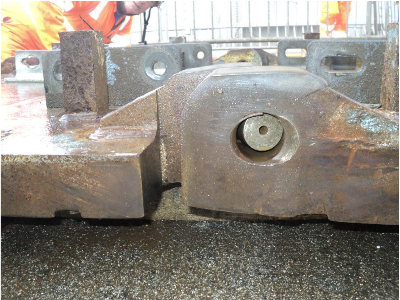
Photograph 13 – Excessive wear on foot and hinge, gap opening between joints.
