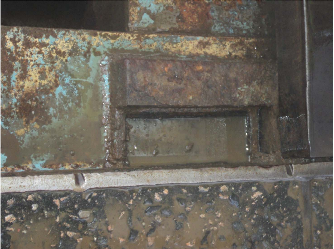
Photograph 9 – Worn lateral restraint at tongue plate and bearing blocks.
