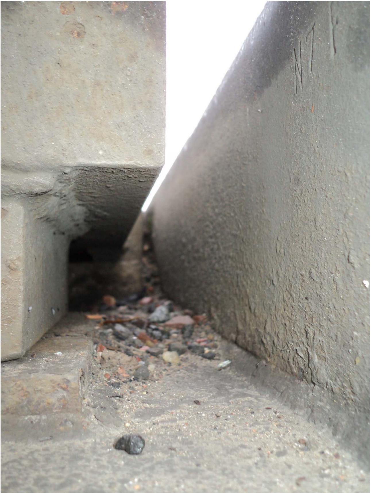
Photograph 18 – Typical debris accumulating at joint.
