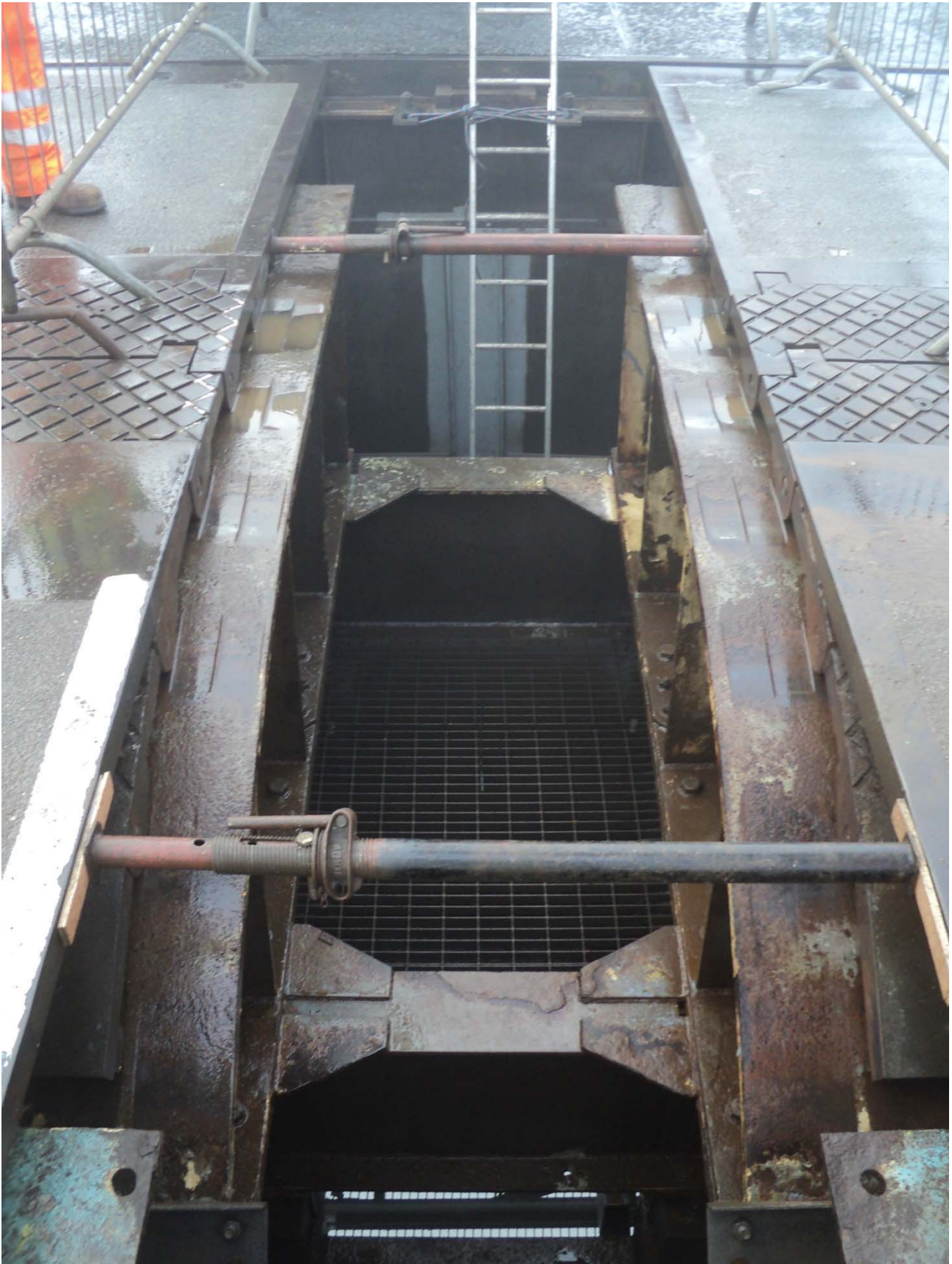
Photograph 10 – General view of slide tracks showing wear at foot locations.
