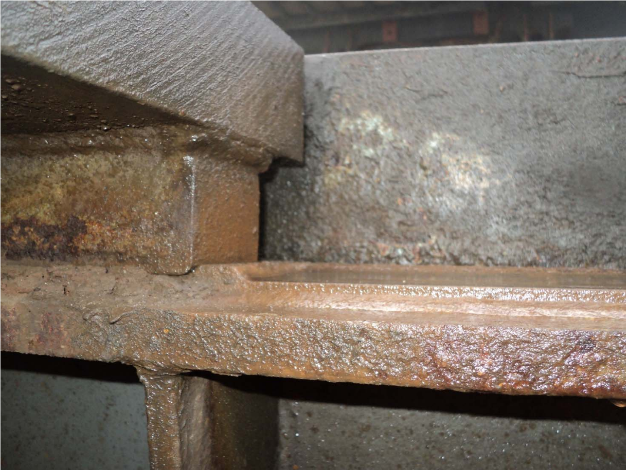
Photograph 16 – Wear in anchor plate support bearings, causing drop in height.
