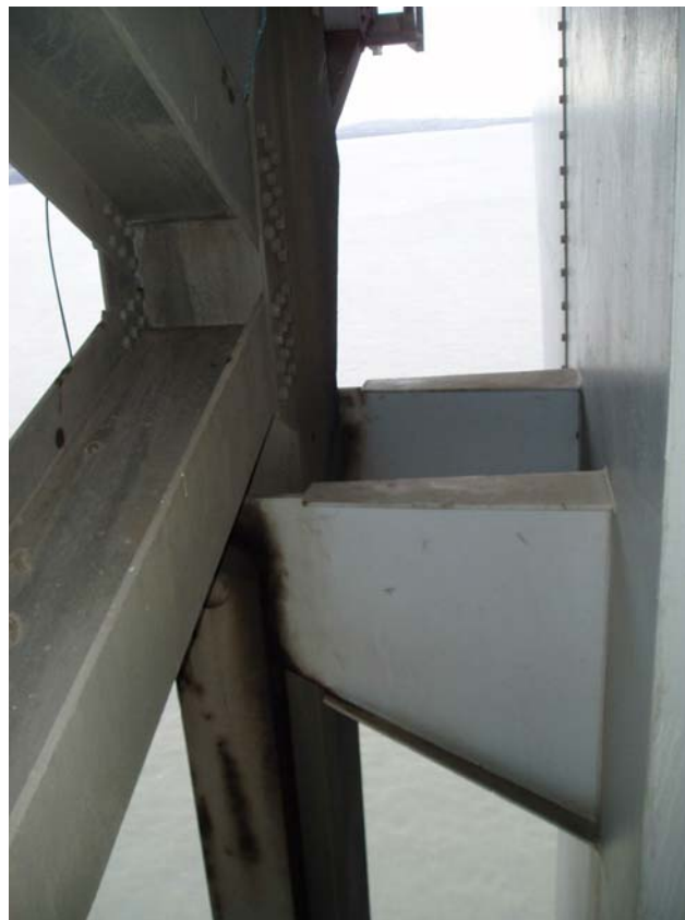
Figure 3 – Main Tower End Link Brackets
