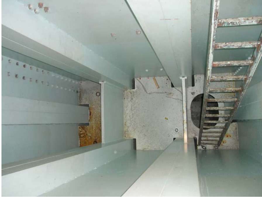
Figure 7 – View on bracket from within the tower, inner cell of the tower is topmost in the photograph
